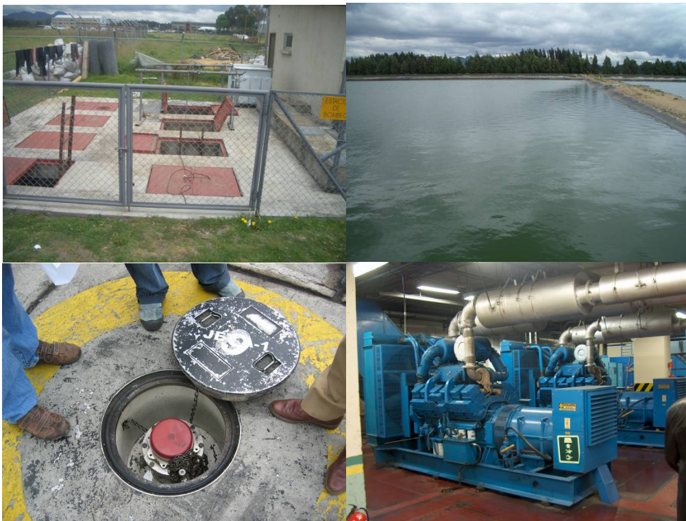
sewage pumping station (t l), facultative sewage ponds (t r), fuel pit (d l), back up diesel generators (d r)
